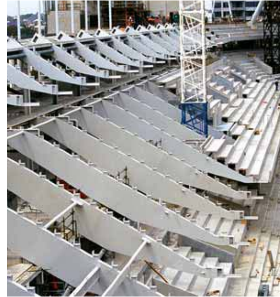
The re-development of Brisbane's Suncorp Stadium relied heavily on XLERPLATE® because it offered a lightweight, flexible design solution.
